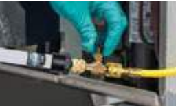
Charge inline with refrigerant
