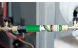
Charge inline with refrigerant
